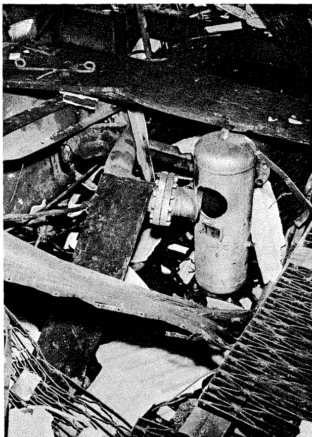
Figure 7. View of 250 lb./sq. in. gauge air separator. Damage to nozzle and outlet line from external force. No internal damage to air system.
